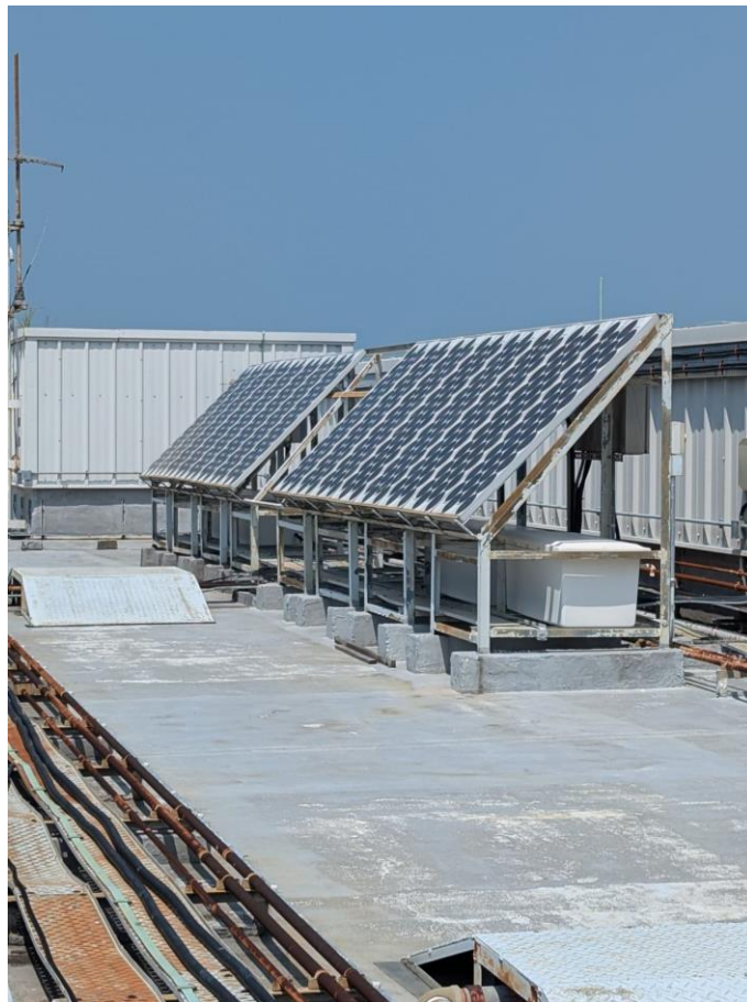
Photovoltaic systems on the rooftop of GFS Headquarters
